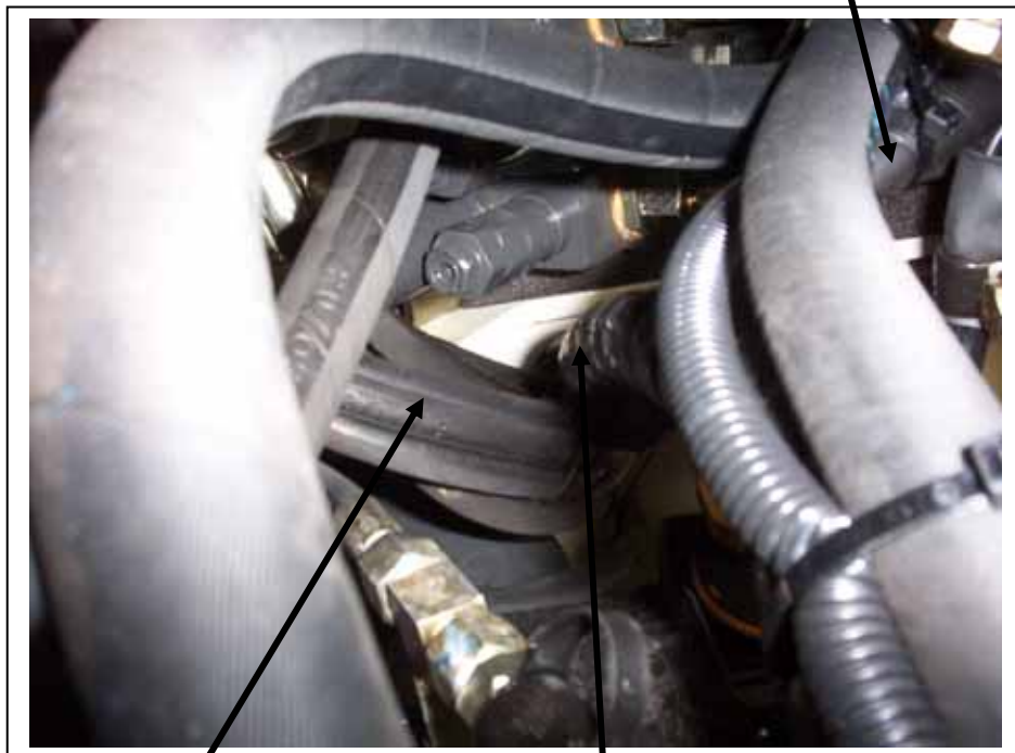
Hydraulic lines running to the underside of the cab
