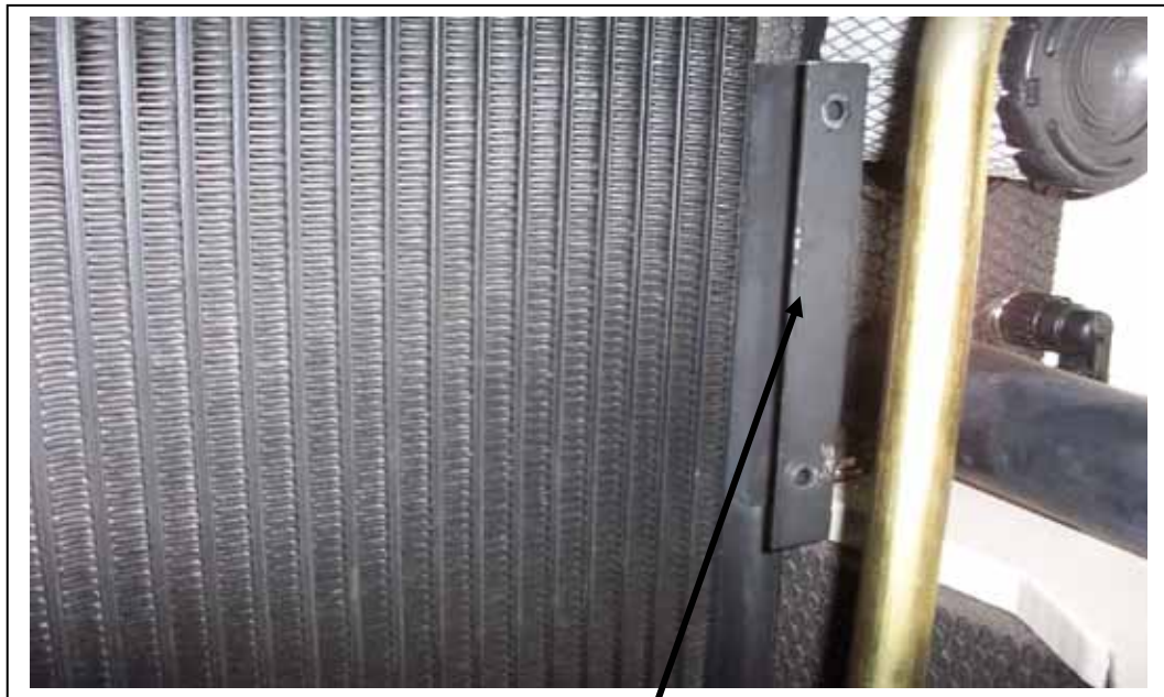
Non fitting side bracket slid between the foam and rad frame and bolted in place.
